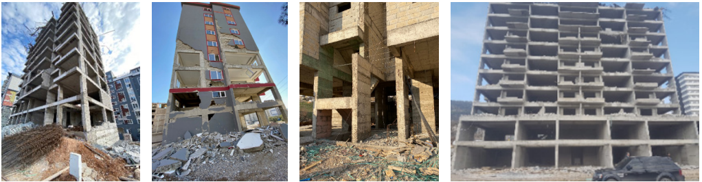
Image 4. Structural and Non-Structural Damage Due to Irregularities in Vertical and Plan Layouts, Including Ground Floor Shops and Mezzanine Arrangements, in Kahramanmaraş After the Earthquake
